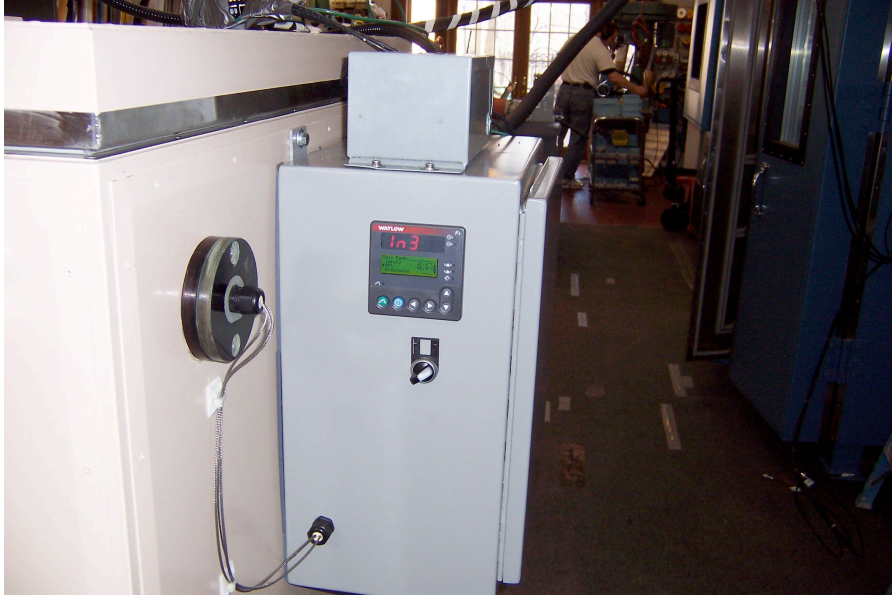
Left Photo Shows front of control counsel. The Controller is a F4S. It also shows the pilot switch and Thermocouples.
