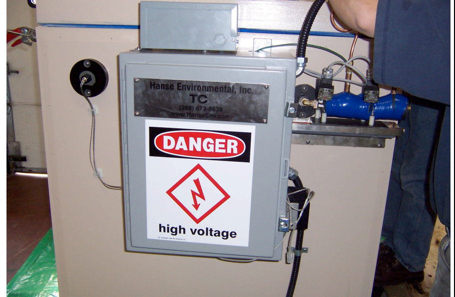
Right photo shows the Ln2 valves and electric council
